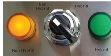
Figure 3-1 Wheelhouse Control Panel
